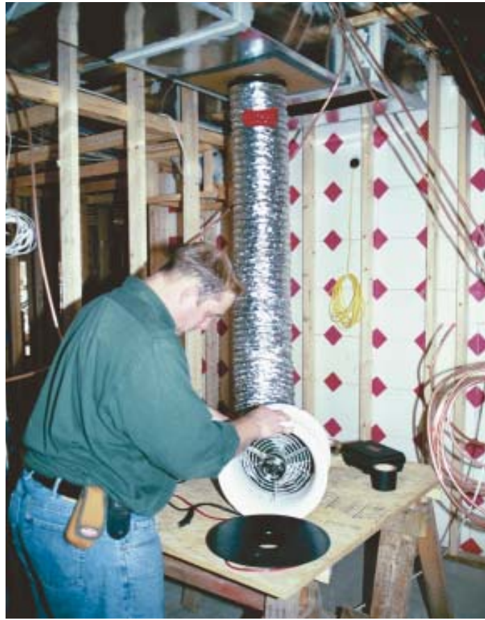
Figure 1. The Minneapolis Duct Blaster is a calibrated variable-speed fan that's tied into the heating or cooling air distribution system at a supply plenum, return grille, or air handler compartment (right). The digital pressure gauge (below) calculates air leakage rates from pressure and fan speed data.
