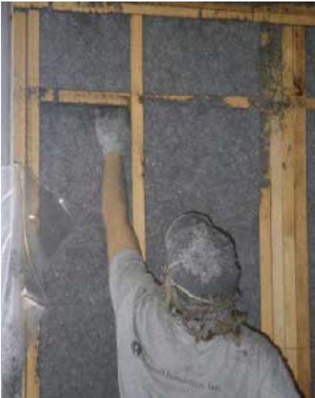
Figure 5. “Smiles” are horizontal gaps that result from poor technique when spraying below window sills, plates, or blocking. To correct the problem, the worker is compressing the insulation by hand before re-spraying the affected area.
