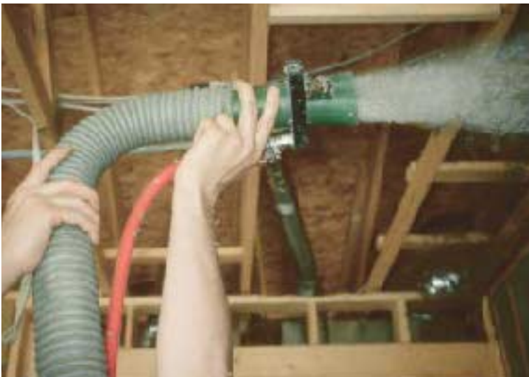
Figure 2. A high-pressure water nozzle moistens both the surface to be sprayed and the insulation as it is blown from the hose. The water flow is adjustable by the operator, who must supply enough moisture to get the insulation to adhere properly but not so much that excess moisture leads to nail pops and other problems. Freshly applied spray cellulose should contain between 30% and 40% moisture by weight.
