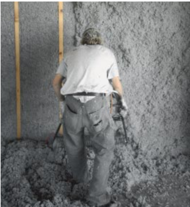
Figure 6. The area at left in this photo has already been scrubbed, leaving the faces of the studs flush with the surface of the cellulose. The scrubbed-off material accumulating on the floor will later be collected, combined with fresh material, and reapplied elsewhere.
