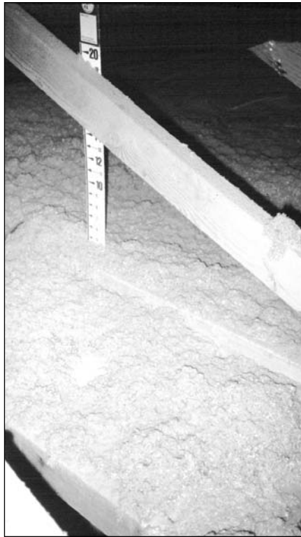
Depth gauges are no guarantee of quality if an installer ignores it, as happened in this attic.
