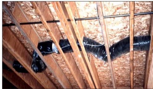
Figure 5. Too many twists and turns in the duct runs create excess resistance to flow. This lowers system performance and can freeze up the evaporator coil.
