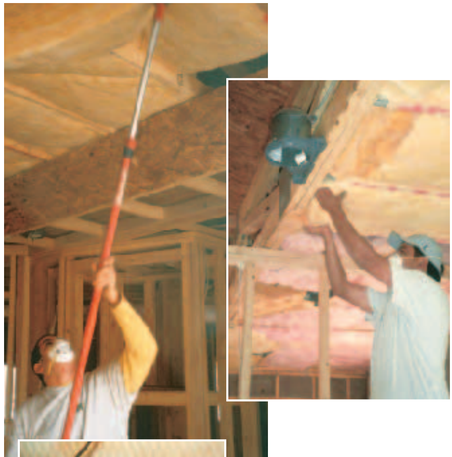
Figure 8. The author’s crew uses toro poles with pronged ends to place batts in high ceilings (left). To reduce convection and infiltration losses, batts should be pulled down to make contact with the ceiling drywall (above).
