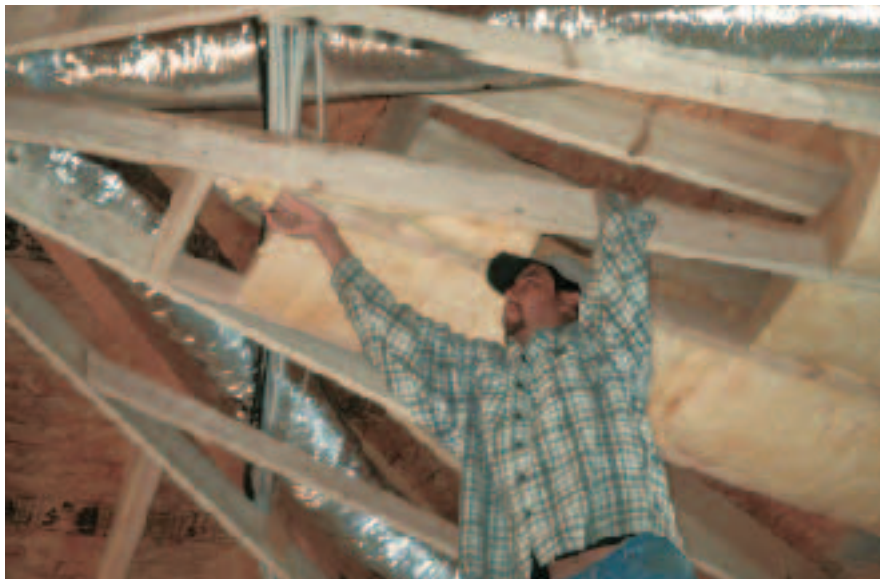
Figure 7. Low “Santa Fe” attics like this one don’t leave room for blown-in products. Instead, carefully fitted batts are installed between the bottom truss chords.
