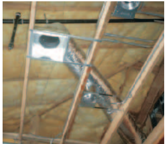
Figure 10. This example of a low-pitch cathedralized attic roof shows how the ductwork is brought within the conditioned space. Batt's fit neatly into the roof-plane cavities, avoiding the need to make complicated cuts and fits around the can lights and other ceiling penetrations.
