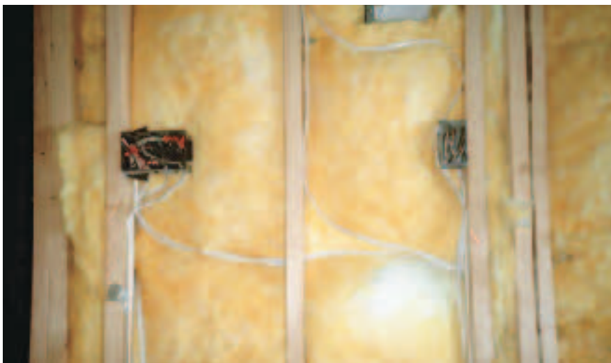
Figure 1. Irregular stud cavities, wiring, and other obstructions in a wall like this make it harder to cut and fit fiberglass accurately. Dark lines and visible stud shoulders in this wall indicate a hurried job.
