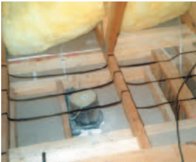
Figure 9. When a dropped ceiling or soffit sits lower than the trusses, the author's crew runs straps between the bottom truss chords to hold the batts in place. This is preferable to a foil or paper support that could fail and let the batts sag, exposing the dropped ceiling to hot or cold air from the unconditioned attic.
